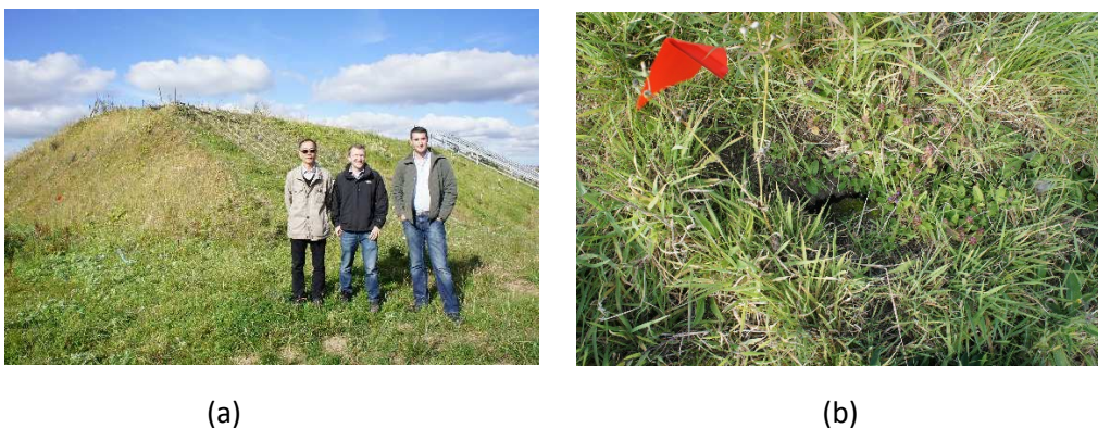
Figure 1. Bionicle experimental embankment. (a) An overall view with my friends Dr Hugues (middle) and Dr Stirling (right); (b) one of the identified cracks
